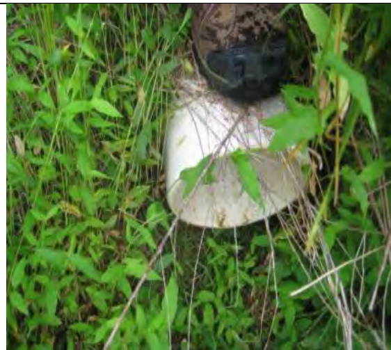
Under drain pipe collects runoff from the bottom of the rain garden and discharges it down-gradient
