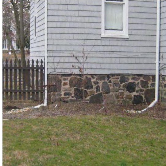
Two downspouts, one rain garden and a large area of conservation landscaping
